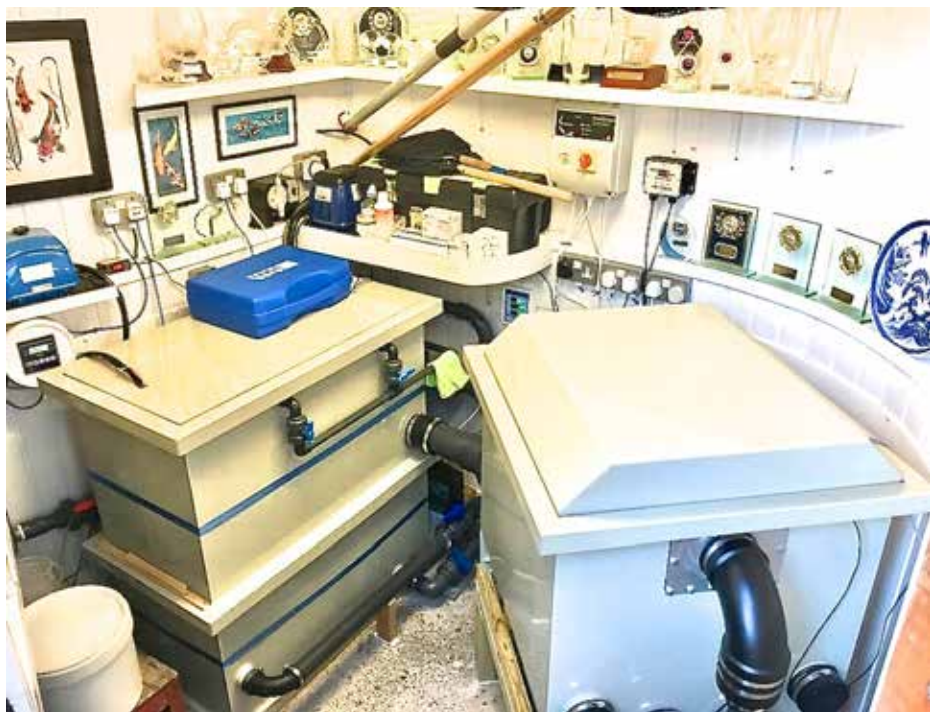
The Filter House with the new drums and all the water testing gear.
