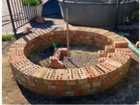
New brick basework is built up to raise level of spawning tanks to allow room for bottom drain pipework.
