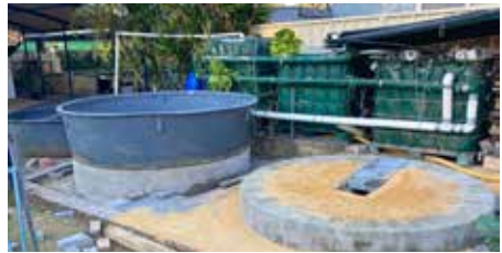
First base complete, right-hand base shows bottom drain connection for pipework ready to connect to spawning tank.
