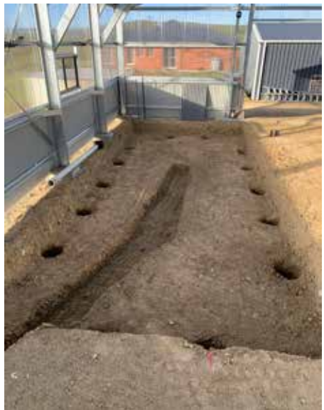
Excavation and pier holes done, ready for the 45,000 L main pond to begin.
