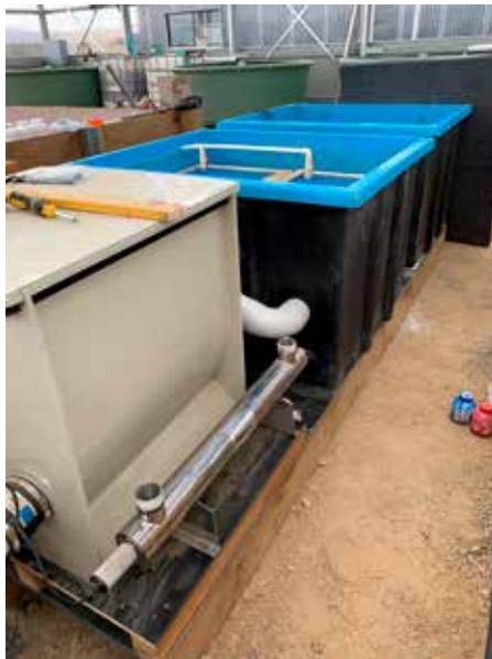
Main pond filtration system almost complete.
